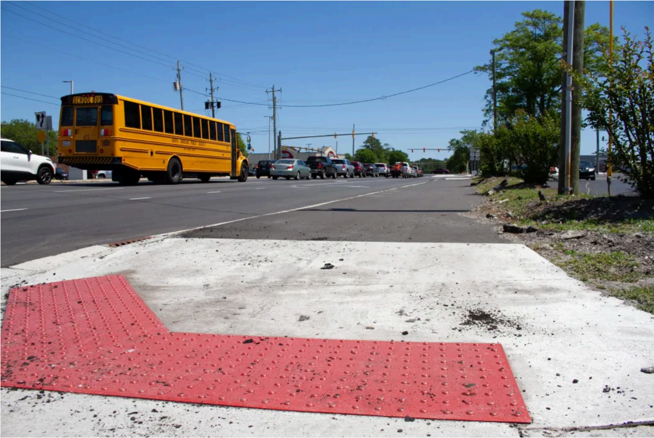
A new curb cut with no separation for pedestrians from the roadway in Wilmington. (Johanna F. Still for The Assembly )
