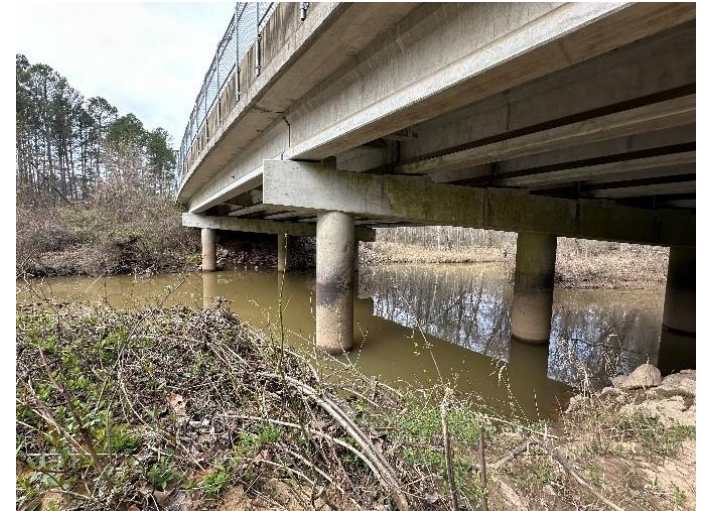
Old Chapel Hill Road at New Hope Creek in Durham County, DCHC MPO
